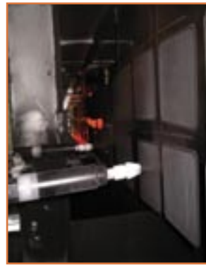
Overhead, conveyORIZED, automated powder coating line with up to 800°F high intensity IR oven
